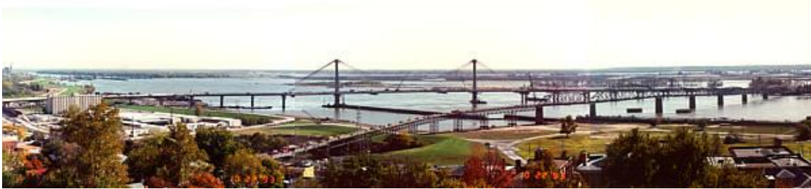
Panoramic view of the new bridges under construction- The Clark Bridge in Alton, Illinois.
